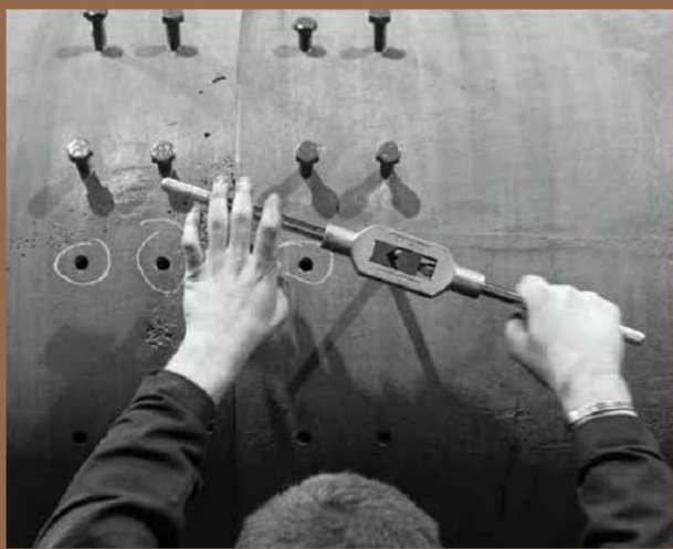
It has taken over two years to painstakingly refurbish the 123 cast-iron gasholders columns
